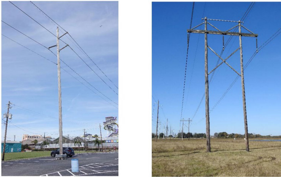
Figure 5-1: Examples of Transmission 138kV Wood Structures
