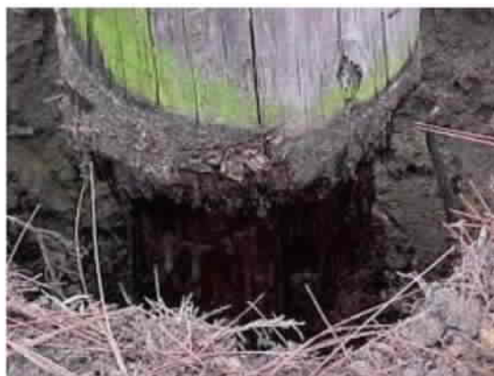
Figure 5 – Below Ground Pole Decay
