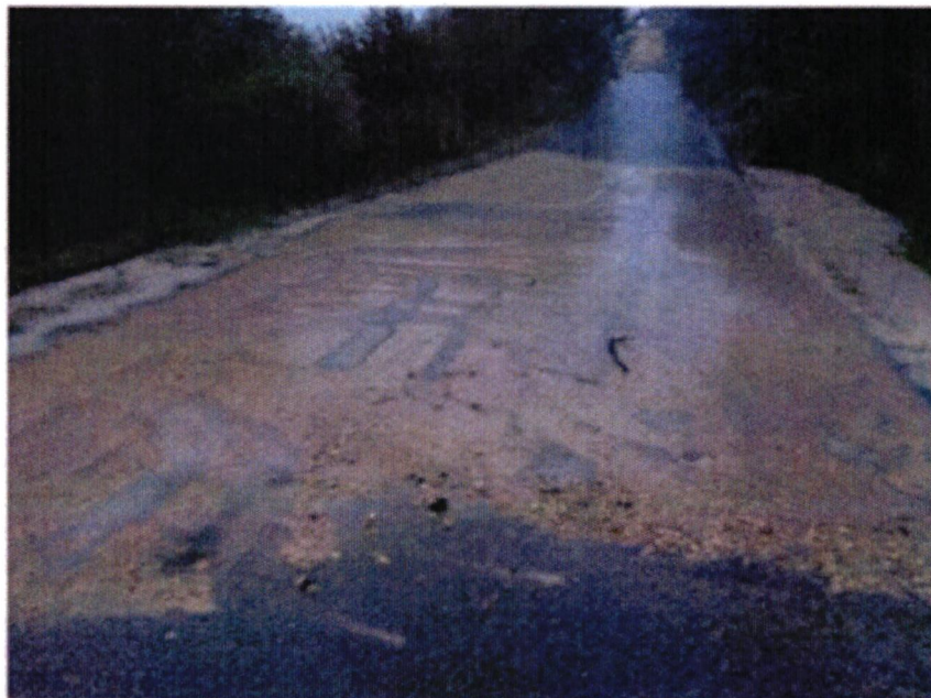
Flooding Over the Altair Road
