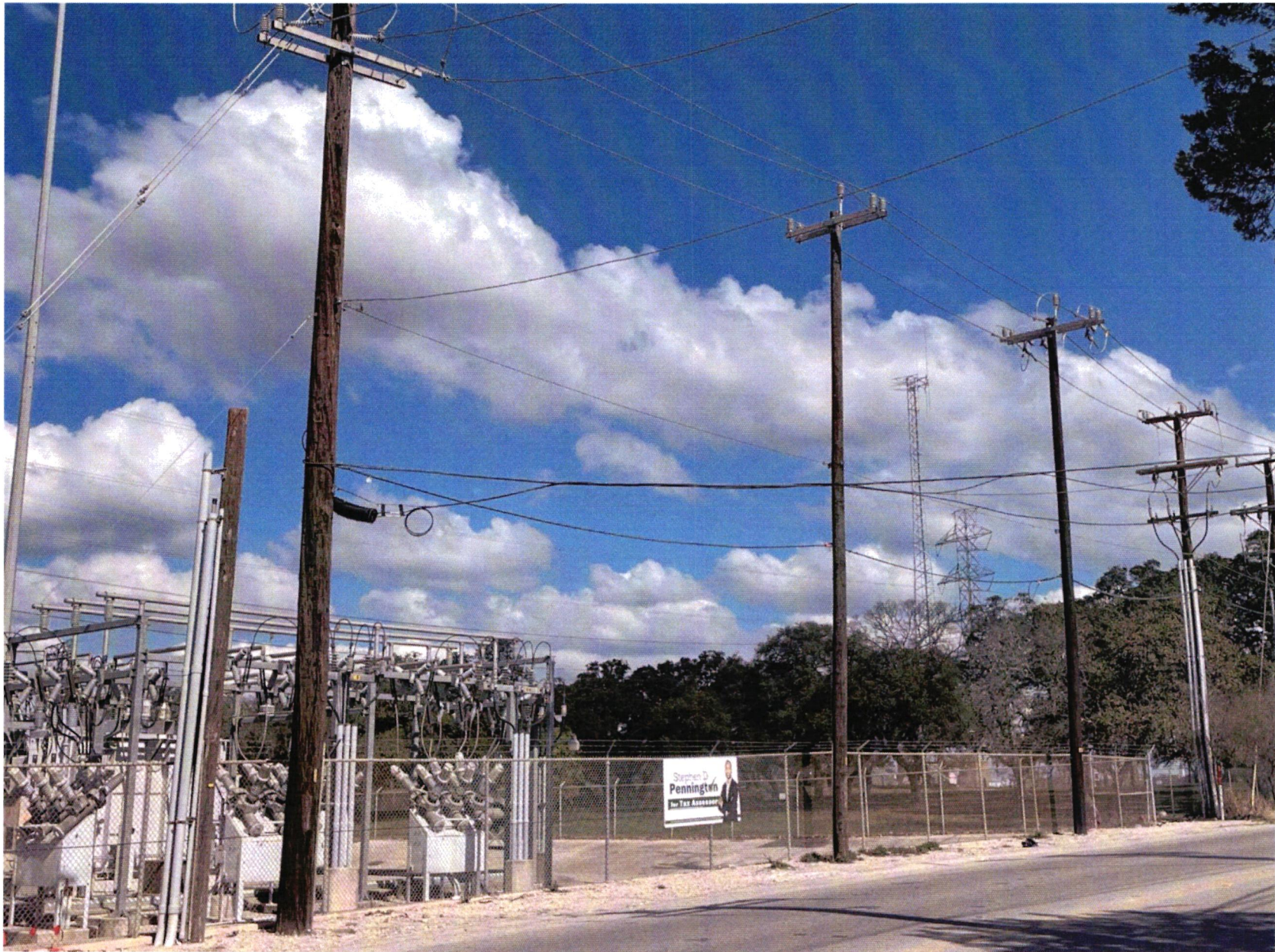
Helotes Substation – March 8, 2021
