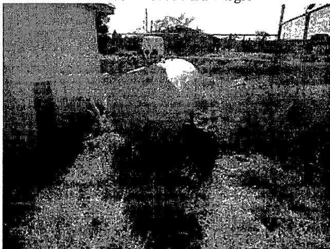
21. Pressure tank Villa Alegre
