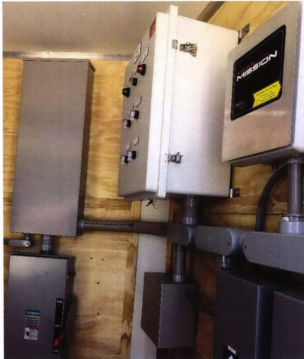
Mobile Pump House Trailer
