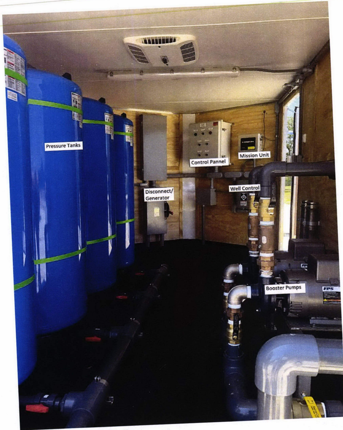
Mobile Pump House Trailer
