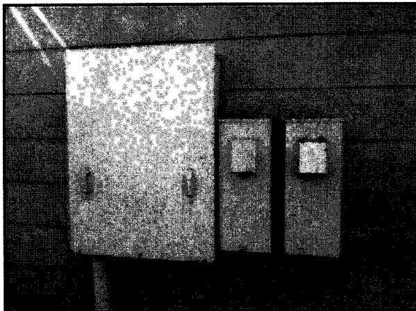
IMG_2226 PWS 1013271 - BOOSTER PUMP BUILDING ELECTRICAL SERVICE RACK
