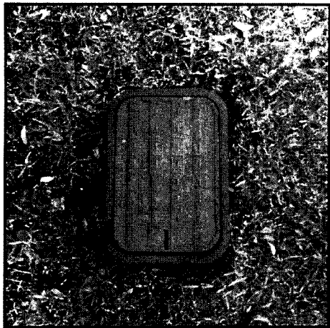
IMG_0932 PWS 1013271 - WATER SERVICE METER BOX
